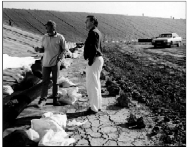
Picture 1. Typical CCL desiccation cracking experienced in hot, dry climates.
