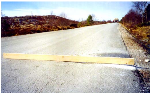
Figure 5 Surface rutting of asphalt overlay, Hitra, Norway
