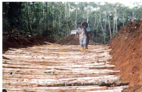
Figure 12 Geosynthetic reinforcement are carried in on an access road of wooden reinforcement
