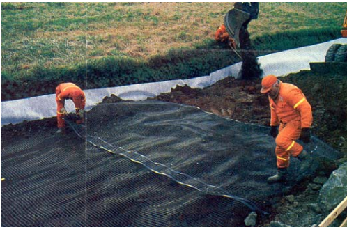
Figure 2 Installation of geogrid reinforcement in a road rehabilitation project in Vesterålen, Norway /3/.
