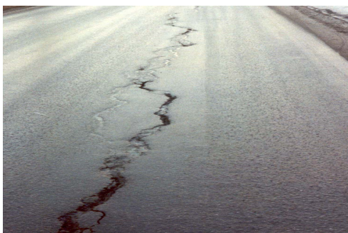
Figure 6 Cracking of overlay due to frost heave, Rælingen, Norway
