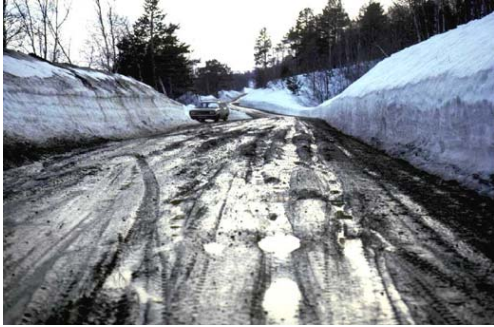
Figure 4 Gravel roads with insufficient bearing capacity, Snåsa, Norway
