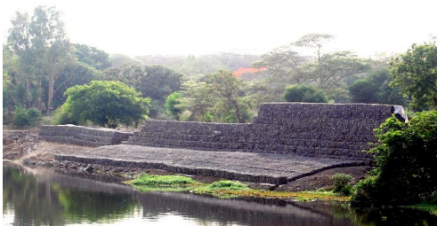
Figure 6. Construction of river bank with Gabions for the Mula river in Pune, India.
