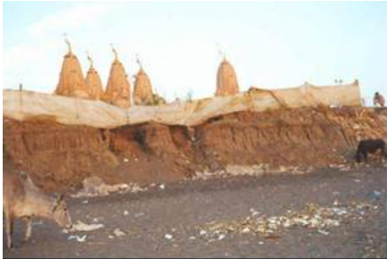
Figure 2a. Eroded shoreline before construction of Gabion wall (Tithal, Gujarat)
