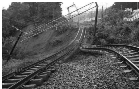
Figure 2. Collapsed earth slope at the Jouetsu-line.
