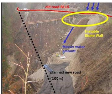
Figure 1. Situation of damaged road
