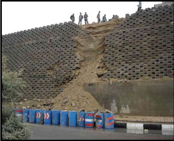
Figure 3. Photo of collapse in the reinforced soil wall
