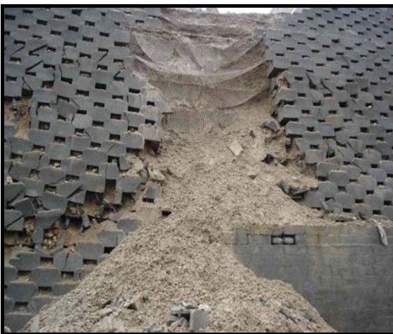
Figure 4. Wall failure-geogrid layers visible
