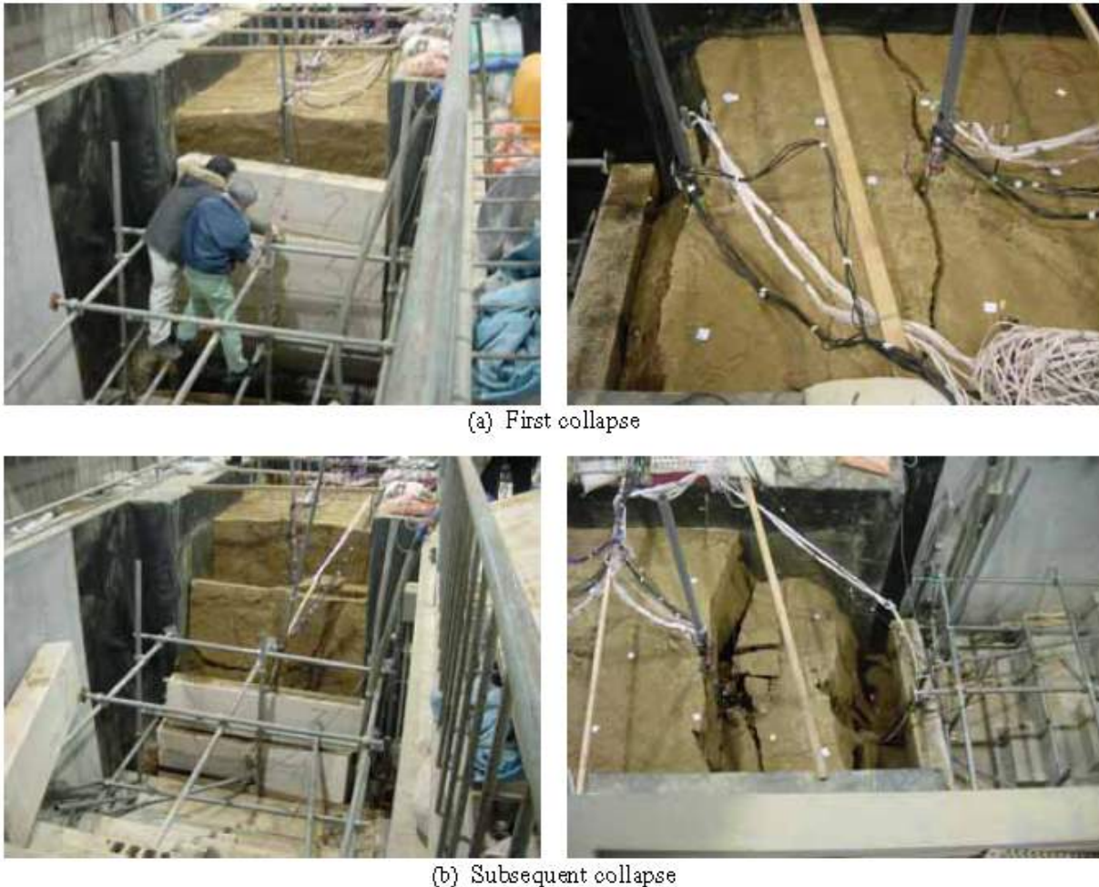
Figure 12. Collapse of case 1 embankment
