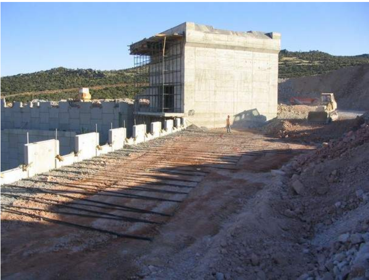
Figure 4. Laying the strips in a zig zag form and spreading the fill.
