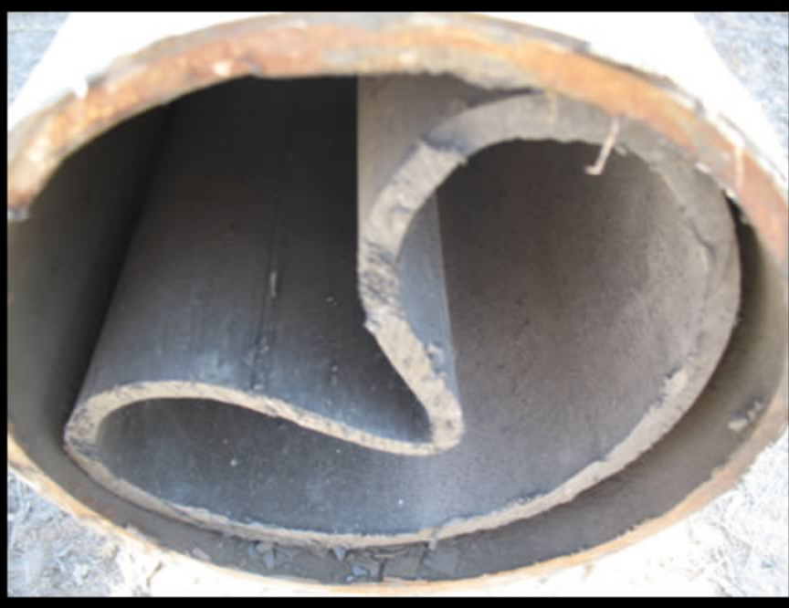
Figure 4. Collapsed HDPE liner
