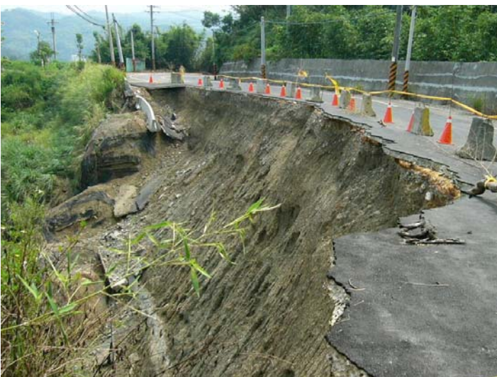
Figure 3. RSS totally collapsed during an attack of typhoon.
