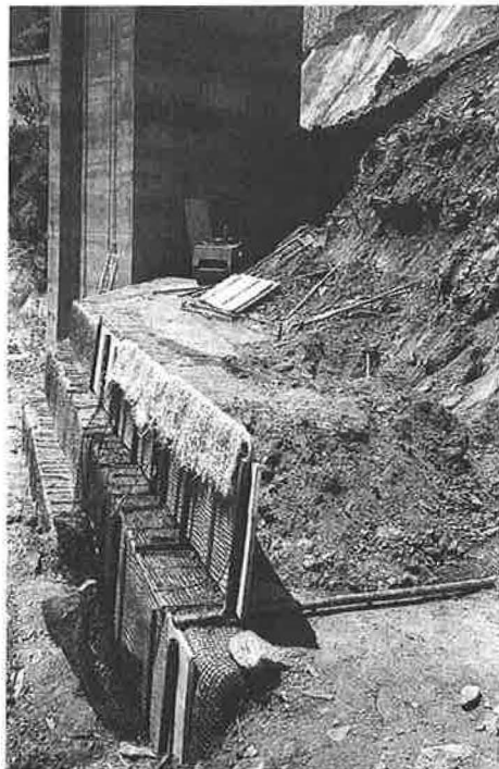
Fig. 2. Detail of the wall during the construction, showing the geogrids, biofelt and the formwork.
