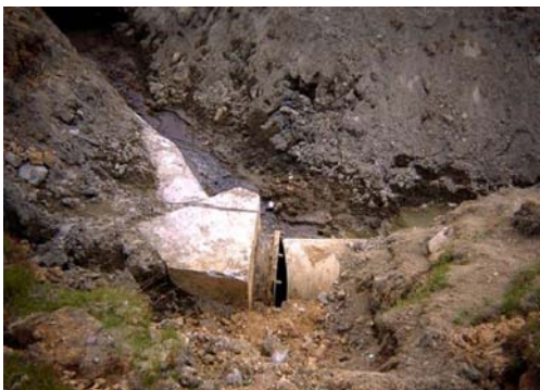
Figure 1. Damage to buried bend in the 1995 Hokkaido-Nansei-Oki Earthquake
