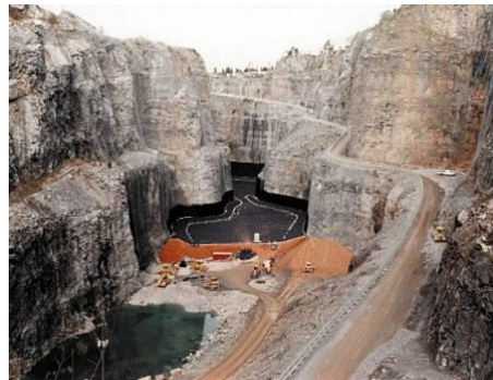
Figure 2 – Geomembrane-lined depleted open pit mine quarry being prepared for solid waste landfill disposal in Virginia, USA in 1998. Reference: Bristol Landfill Photo (1997), www.bristolva.org/WasteDisposal , Bristol, Virginia.
