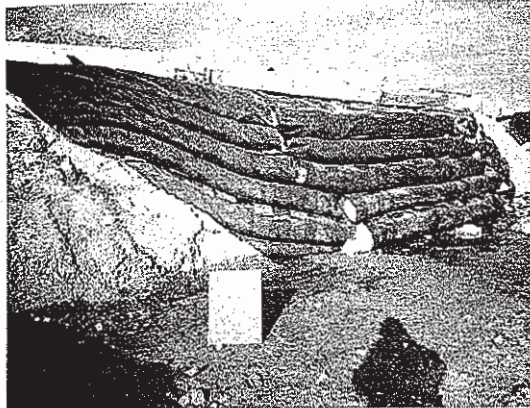
Photo 4 Failure pattern in Section 2
