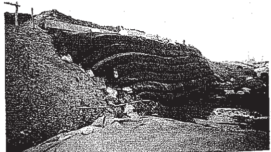
Photo 3 Failure pattern in Section 1
