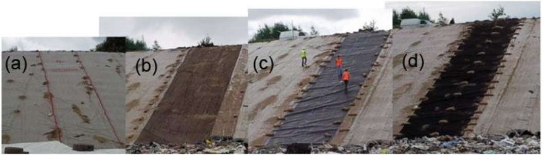
Figure 1. Stages of materials deployment Milegate July 2009: (a) original geotextile liner; (b) uncovered clay layer; (c) geomembrane liner; (d) geotextile protection liner.
