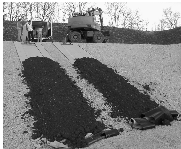
Figure 3. Laying down the protective soil cover on the slopes of a motorway basin
