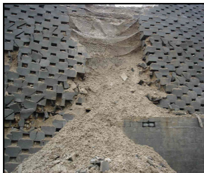
Figure 3. Wall failure-geogrid layers visible
