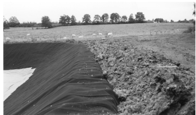
Figure 13. Fastening of a geocomposite drainage layer at the head of the embankment
