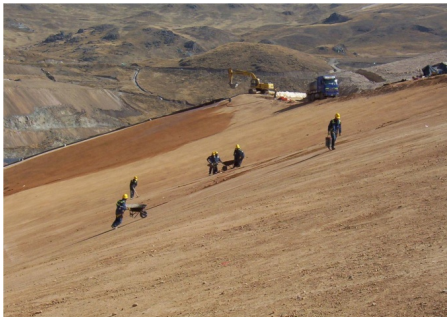
Figure 2: Very steep slope for a leach pad.
