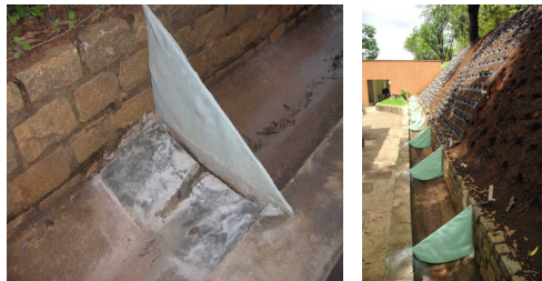
Figure 4 - Detail of the partition wall and overview of the drainage channel fitted with all divisions of parcels.
