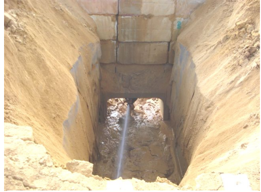
Figure 5: Undermined from below, the sides of the resultant trench were close to vertical
