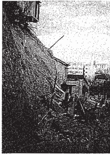
Fig. 29 A collapsed masonry wall located near the Terre Armee wall TA2 (JTAA, 1995)
