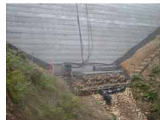
Fig. 5. Final treatment of drain water
