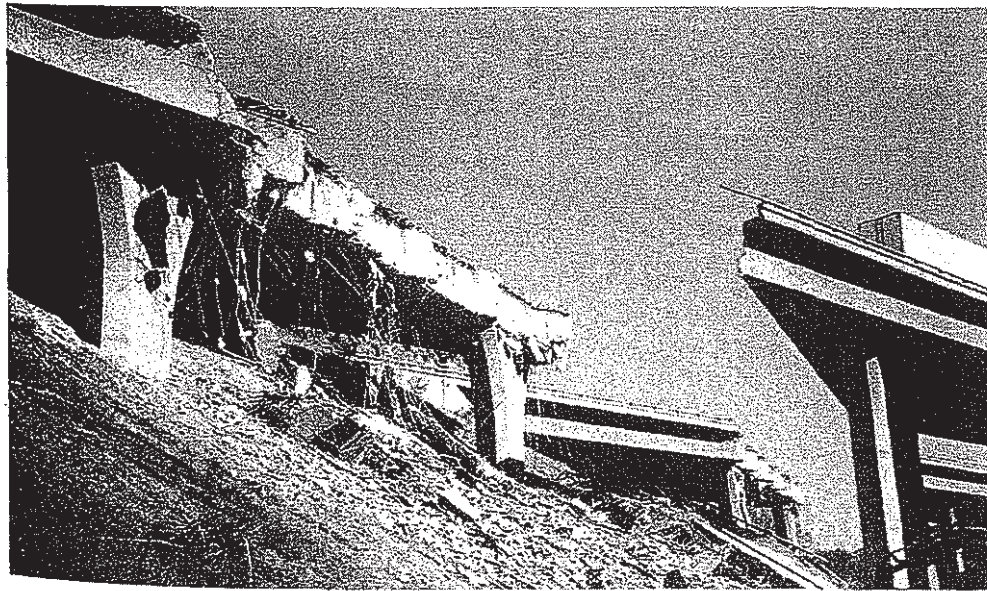
Figure 1. Collapsed Bridge on Interstate 5 at Gavin Canyon 2 km from Lyons Avenue Reinforced Earth Wall (Civil Engineering, March 1994)
