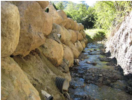
Figure 4. Drainage tubes passing through the boulders bank of torrent.
