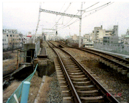
Picture 1. The damage of bridge abutment at Hyogoken-Nambu Earthquake (1995.1.17 M=7.2 Kobe)
