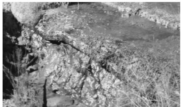
(b) Clogged geotextile.
