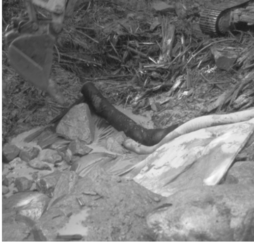
Figure 2. Routine application: placement of riprap stone over the geotextile for streambank stabilisation.
