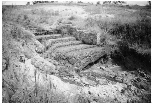
(a) Collapse of the channel.
