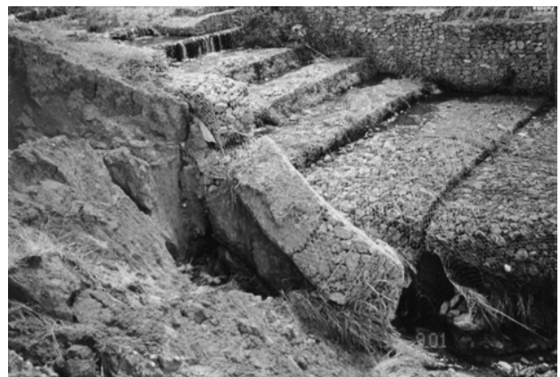
(c) Erosion at the channel side wall due to lack of filter.
