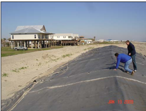
Figure 1. "Geo-burrito" Grand Isle, Louisiana. A woven geotextile was used to wrap a clay core to provide emergency protection.
