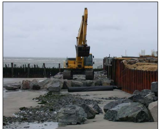
Figure 2. Use of geotextile separation fabric under stone toe fronting a steel sheet pile bulkhead, Strathmere, New Jersey.
