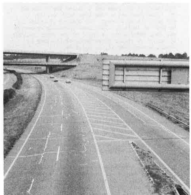
Fig. 5 Cracks demarcated with Lime during a Survey February 1982
